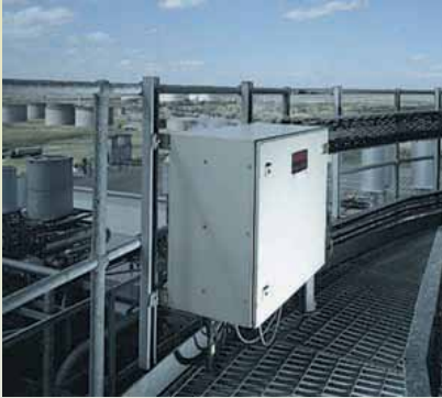
Installed LAND FGA
