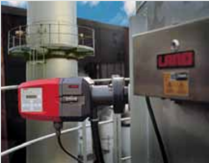
Installed Model 4500 MkII+
