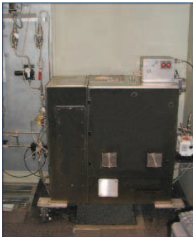
Figure 2: AMETEK ProMaxion Process MS in GMH analyzer shelter
