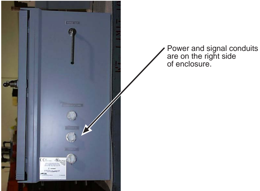
Figure 5: Power and signal conduits
