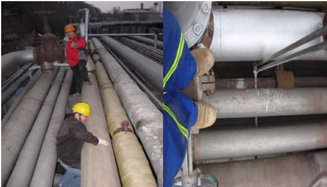
Fig. 3. Example of Accessing a Difficult Tail Gas Analyzer Sample Point.
